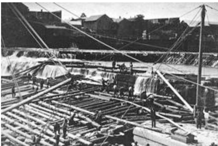
St. Paul photographer C. A. Zimmerman captured this view of workmen building a wooden apron below the St. Anthony Falls to prevent further erosion of the limestone in 1870. (MN Historical Society photo)
